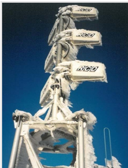
Antennas of TETRAPOL Radio System
